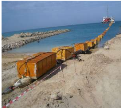
Petronas Turkmenistan (Various Pipelines)
