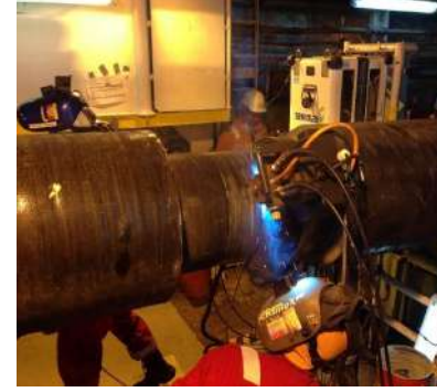
Lukoil Caspian (Various Pipelines)
