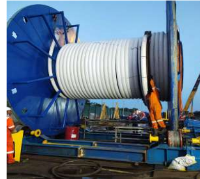
Brunei Shell Salman (Flexible Pipeline)
