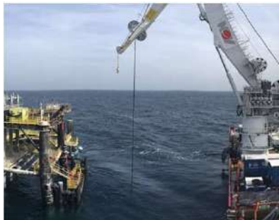
Qatar Petroleum NFA (Various Pipelines)
