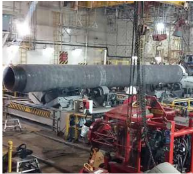
Petronas SK316 (Pipeline)
