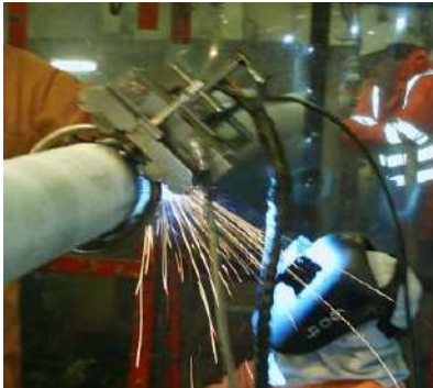
Shell Ormen Lange (MEG Pipeline)
